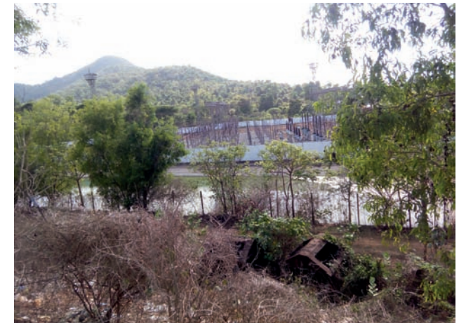
Leachate storage tank at the Karwar landfill site
