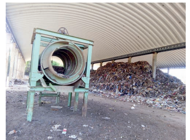
Waste compactor installed at the Karwar landfill site
