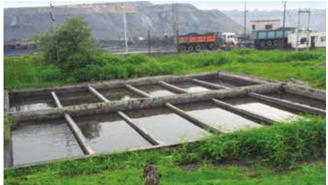
Primary settlement tank inside the mine
