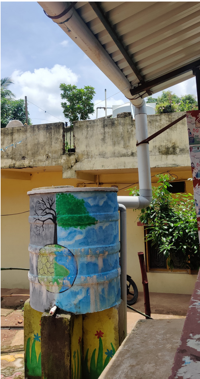
Figure 23: Rain Water Harvesting Structures
