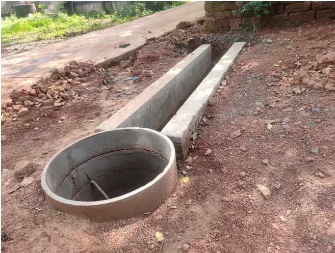
Figure 22: Rain Water Harvesting Structures
