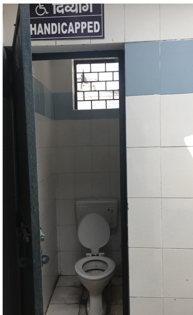
Photo 9: Handicapped toilet in new CTC in Mangolpuri without handrails
