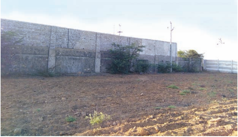
Wall surrounding the back of the company raised to 9 m after the complaint. Pic: Hasmukh Dhumadiya
