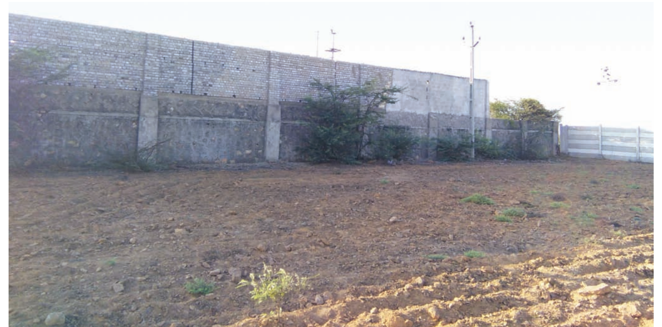
Wall surrounding the back of the company raised to 9 m after the complaint. Pic: Hasmukh Dhumadiya
