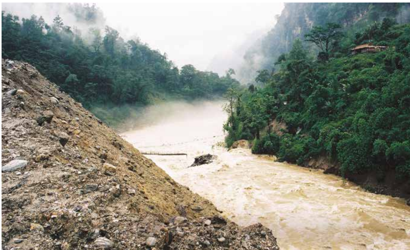
Muck dumping in the Teesta River due to construction of a hydropower dam
