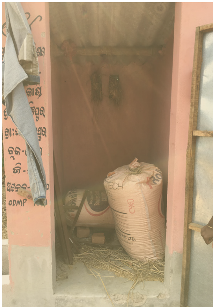
Unused toilet facility being used for storage in Puri
