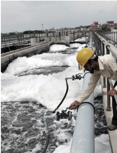
Sewage treatment plant in Delawas, Jaipur. source: Asian Development Bank
