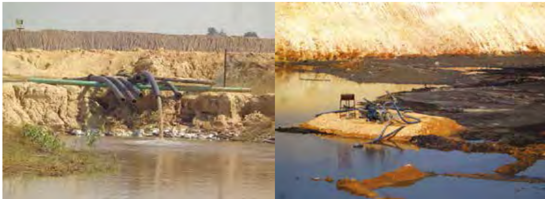
Dumping of waste water from the coal pit via a motor and pipeline
