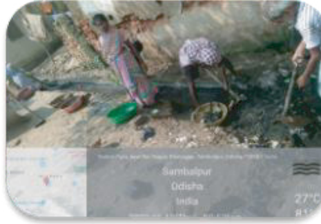
Storm Water Drainage
