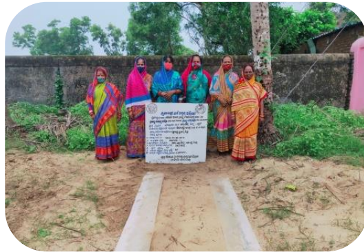
RAIN WATER HARVESTING STRUCTURE
